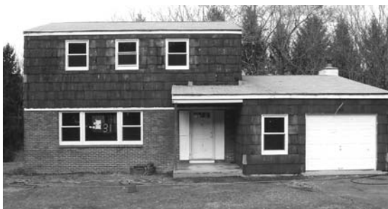
The three additional houses in the CHAMP Program as they were being renovated.
